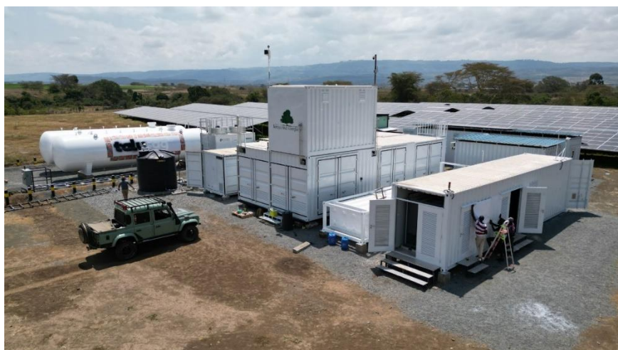
Figure 18 - The ammonia plant at Kenya Nut (Source: Talus Renewables)
